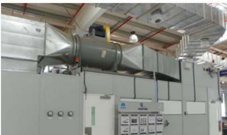
Model QSL Spray Paint Booth Exhaust
