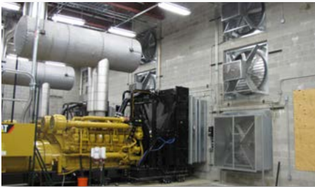
Model WPB Generator Room Exhaust
