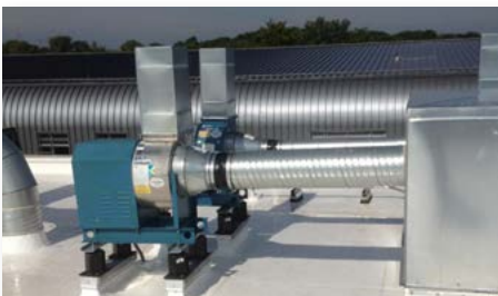
BCV Building Exhaust
