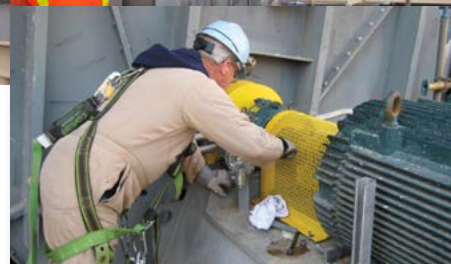
Coupling & Sheave Alignment
