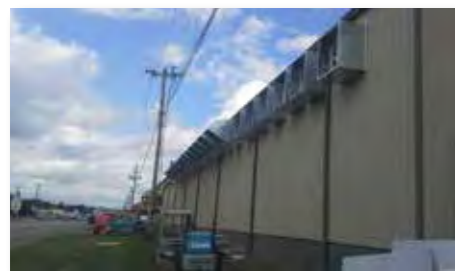
WPD Warehouse Exhaust
