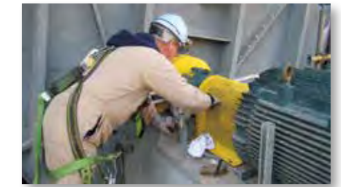
Coupling & Sheave Alignment
