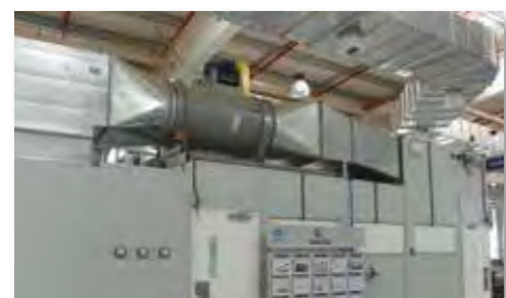
Model QSL Spray Paint Booth Exhaust
