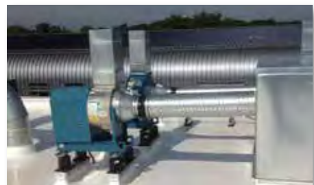
BCV Building Exhaust
