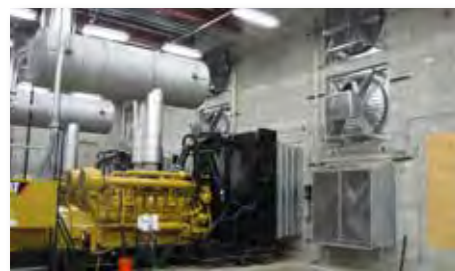
Model WPB Generator Room Exhaust
